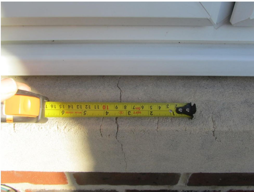
Photo 5 – View of cracking which has become wider than hairline cracking width.
