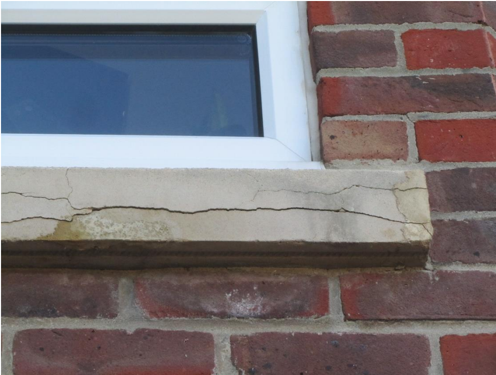
Photo 2 – View of a previously repaired and decorated cill that is now experiencing large cracking. Typical category 1.
