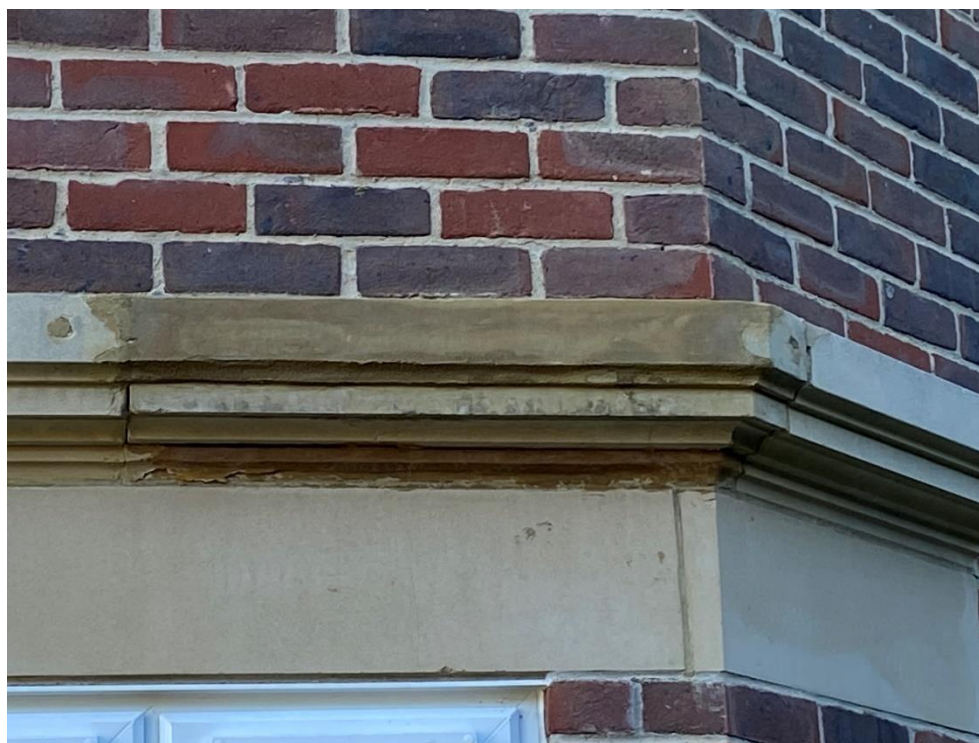
Photo 6 – View of poor repair to string course above window head to the rear elevation.
