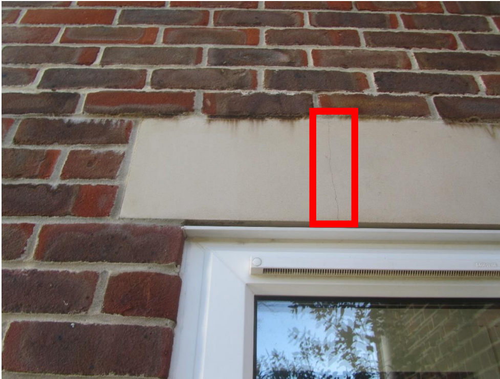
Photo 4 – Typical view of hairline cracking to head. Typical feature of a category 3.
