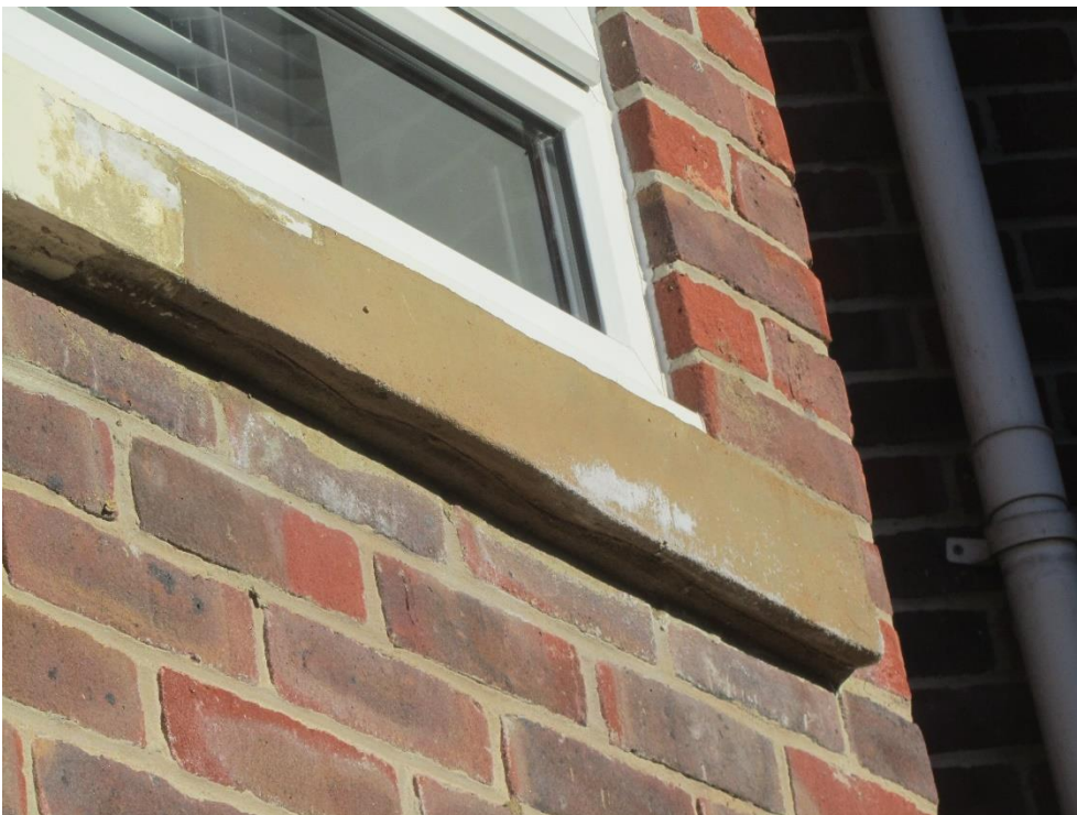
Photo 3 – Cill which has had an historic repair and decoration. This is typical of a category 2 as it has potential to worsen over time. It is also at first floor level.
