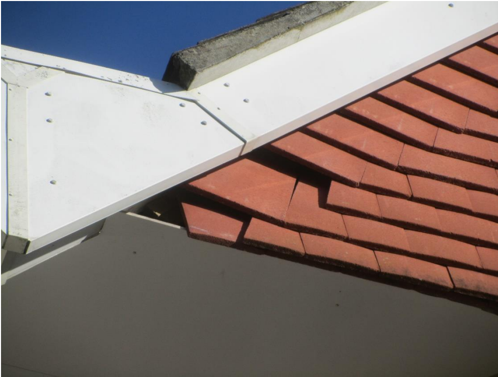
Photo 8 – View of slipped tile hanging to the front elevation gable.
