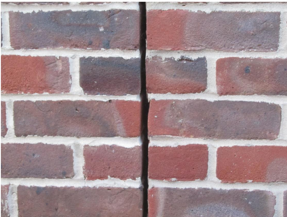
Photo 10 – View up close of expansion joint, showing no filling inside the joint.
